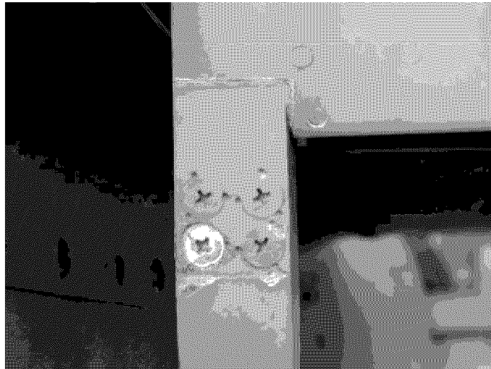
Fig. 10 – Galvanic Corrosion on the MB-339 between Mg Alloy Trim and Aluminum rivets
