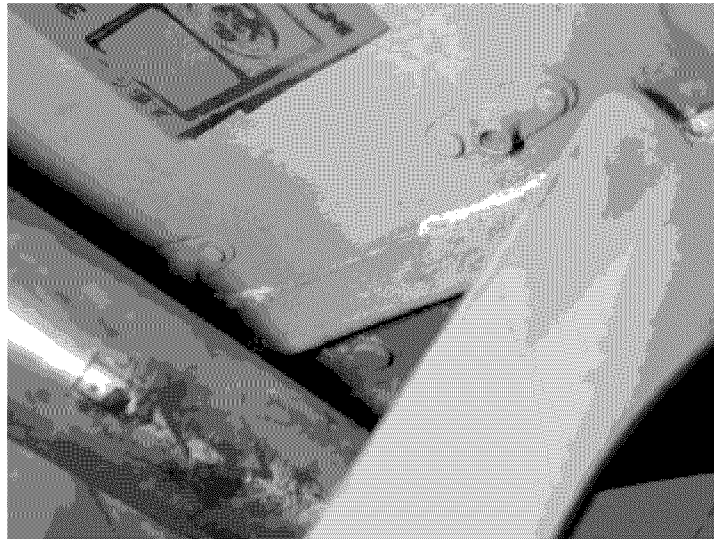
Fig. 11 – Galvanic Corrosion on the MB-339 Attach Fitting
