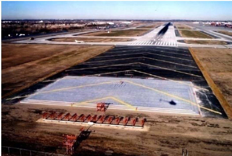
Figure 13: An EMAS bed installed at Minneapolis-St Paul International Airport (KMSF), runway 12R end
