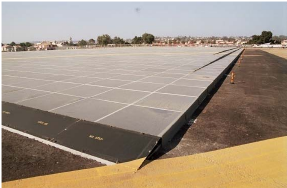
Figure 14: An EMAS transition ramp at San Diego International Airport (KSAN), runway 09 end
