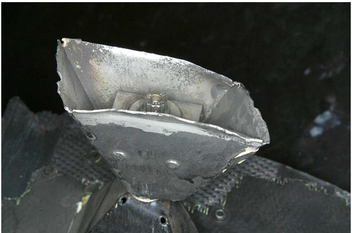
Figure 12. Base of a bolt tower illustrating the failure and separation from the flange transition.
