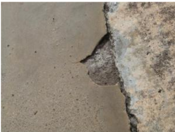
Example of Failed SRE Repair (where the material was too thin)
