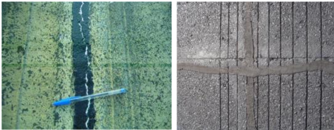
Examples of Poor Rubberised Bitumen Banding
