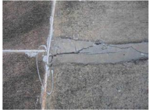
Example of "Poor" Concrete Repair
