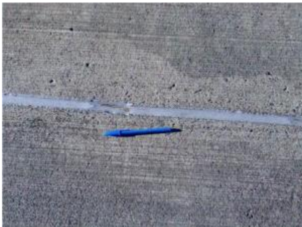
Example of Good Joint Sealant
