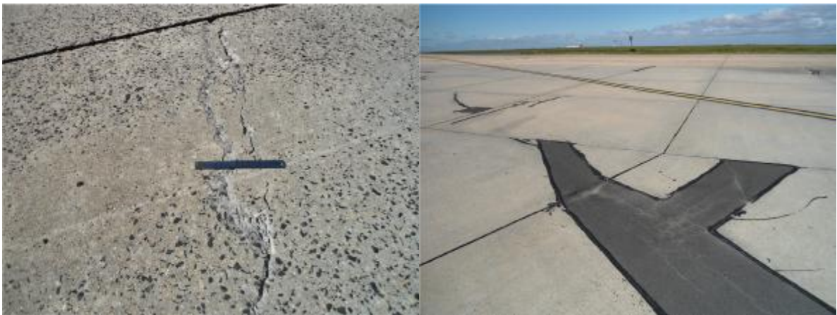
Examples of Cracked Concrete Pavements and Repaired Pavement Requiring Repair
