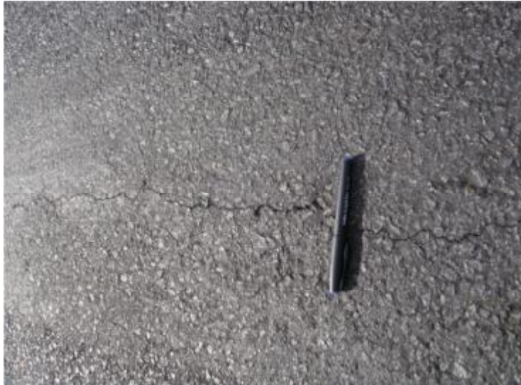
Example of Low Severity Cracking
