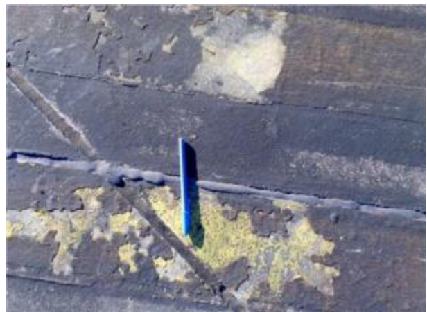
Example of Poor Joint Sealant
