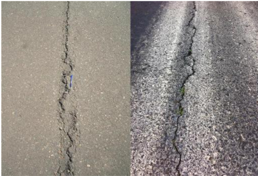
Examples of Severe Reflection Cracking in Asphalt Pavements
