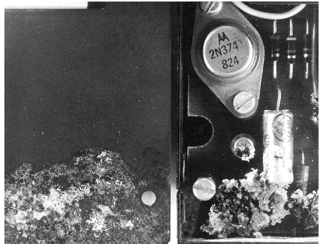
Figure 3-1. Corrosion Caused by Blown Capacitor Acid
