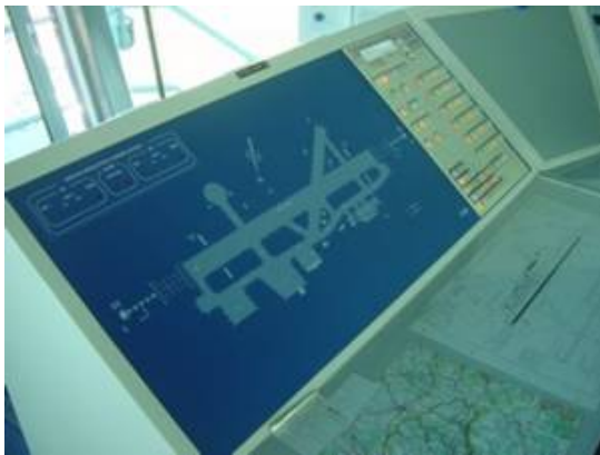
Luxembourg Findel Airport Lighting control panel
