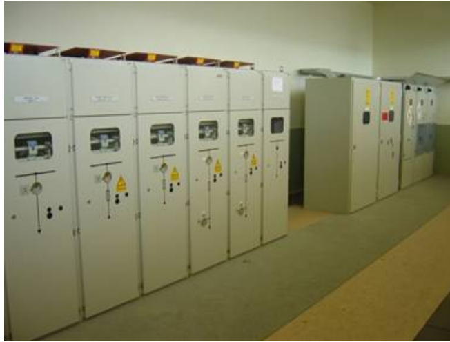
Luxembourg Findel Airport - Medium voltage distribution cabinets
