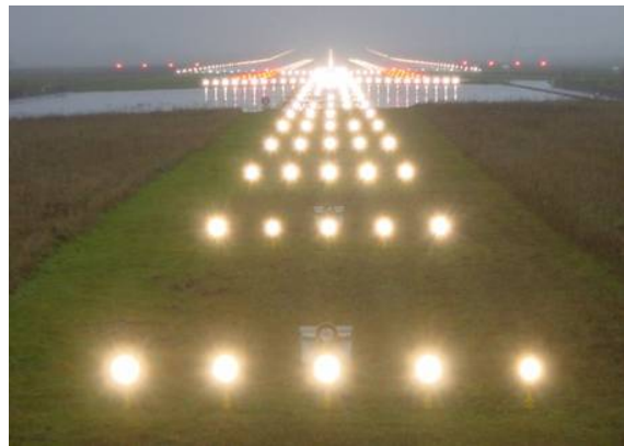
Approach lighting Luxembourg Runway 24
