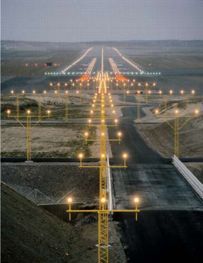
2.1.2 (Below) AWOPS Runway with Calvert & Supplementary Approach Lighting in last 1000 feet
